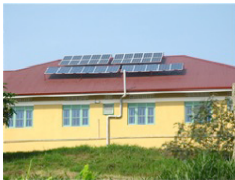
Solar panels on KIDA's new hospital building
